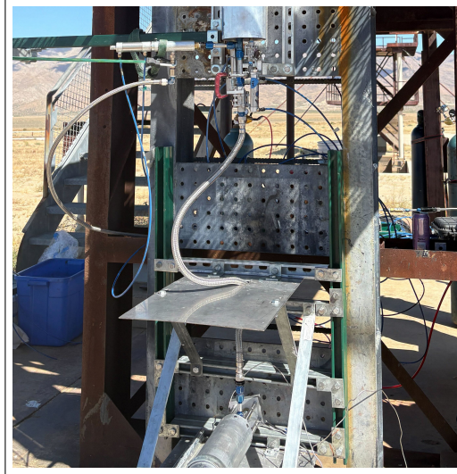
Figure 3: Non-optimal flex hose with excessive bends
